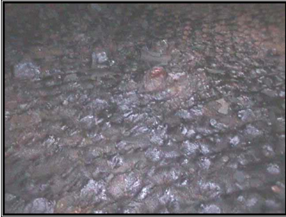
Example of Fouled Dual Flow Tray
